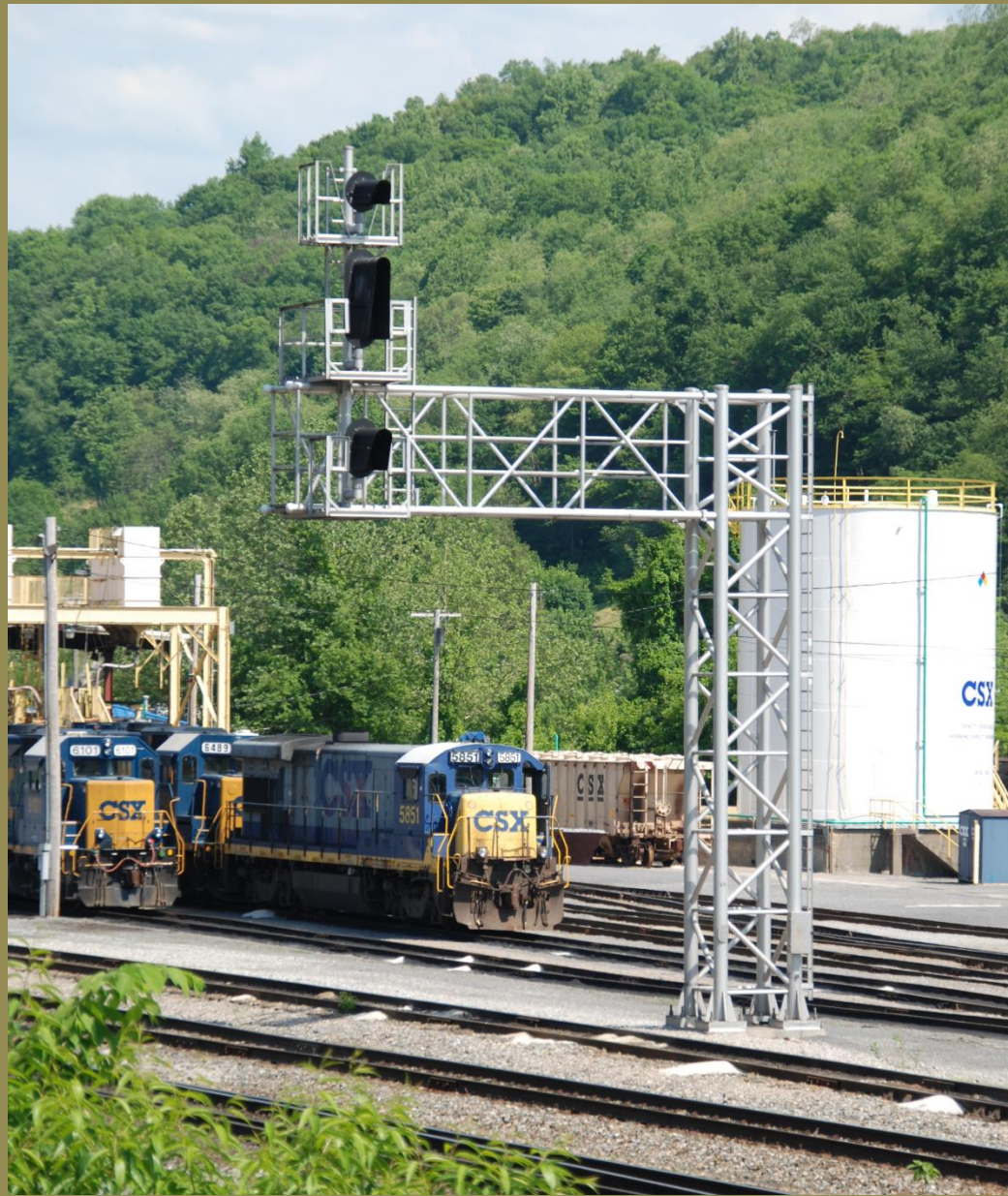
New “Darth Vader” color light signals new style signal “mast” CSX, Grafton, WV - Replaced B&O CPL’s
